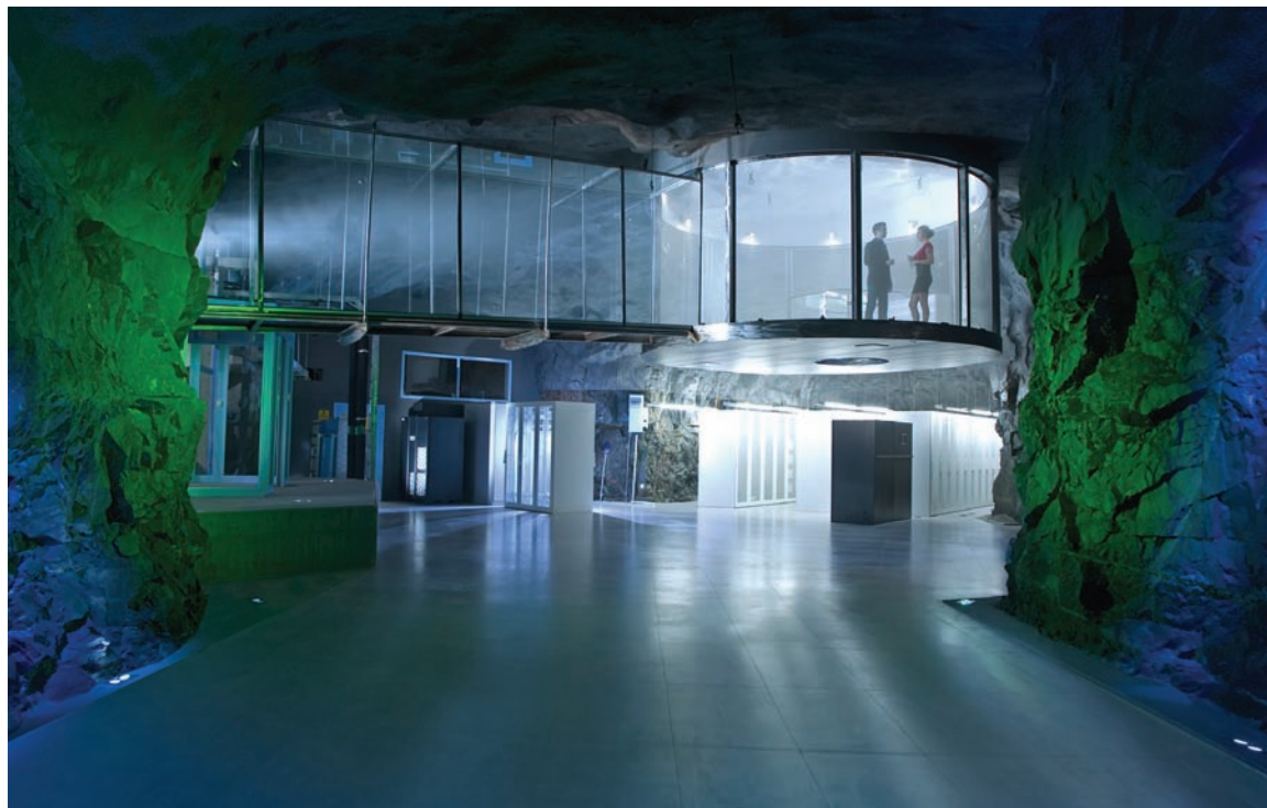
FIGURE 3-3 A circular, glass-walled conference room overlooks the Bahnhof Data Center's server rows.
