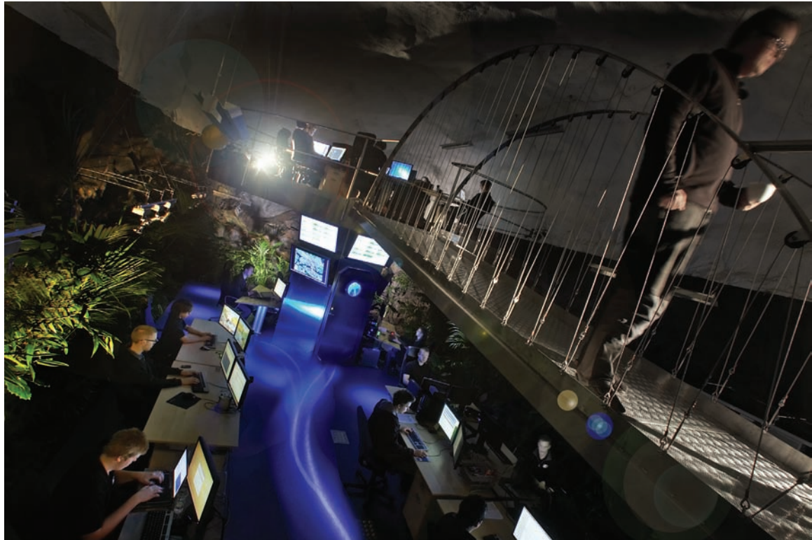
FIGURE 3-2 The Bahnhof Data Center's Network Operations Center (NOC). Artificial daylight, greenhouses, and even a saltwater aquarium have been installed to avoid the impersonal feel of many conventional Data Centers.
